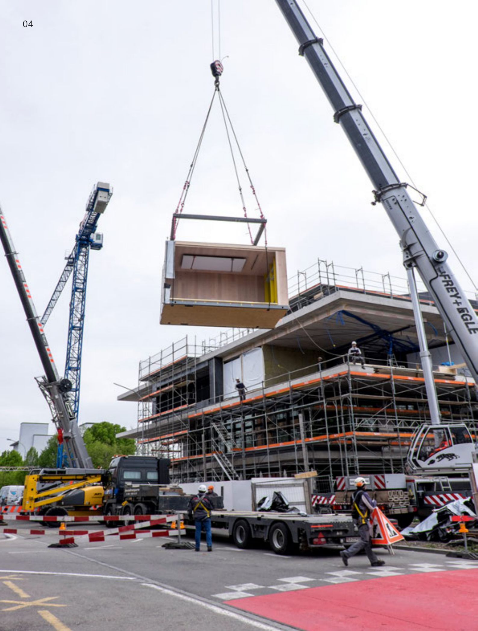
Installation of the prefabricated modules for the Vision Wood unit on April 26, 2016.
