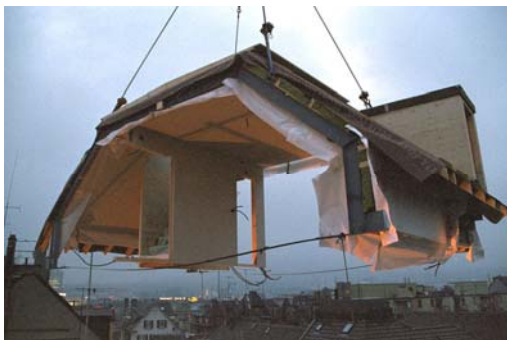
The prefabricated roof module during the renovation of a model building, Magnusstrasse, Zurich (Architect: K. Viridén, Zurich).
