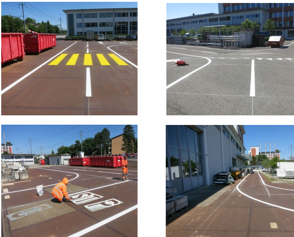
Figure 21: Upper left: Test track stop intersection with zebra crossing Upper right: Yield intersection. Lower left: Painting the stop marking. Lower right: Single-lane back straight
