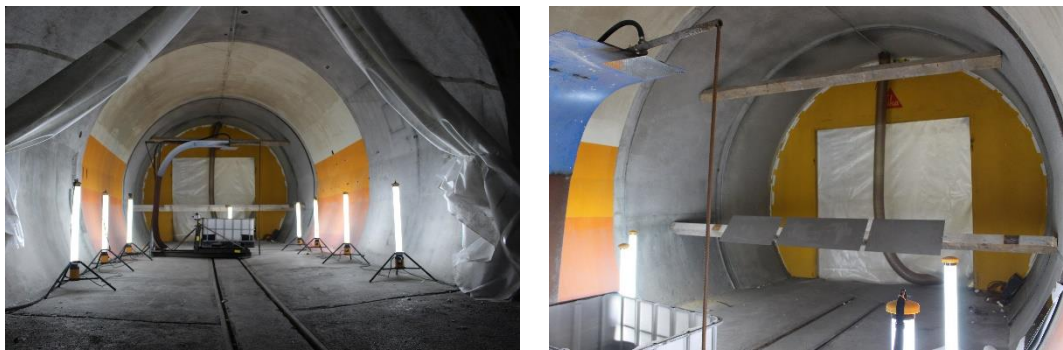
Figure 8 Testing site tunnel 'A' (left) with exhaust air purification equipment (right)
